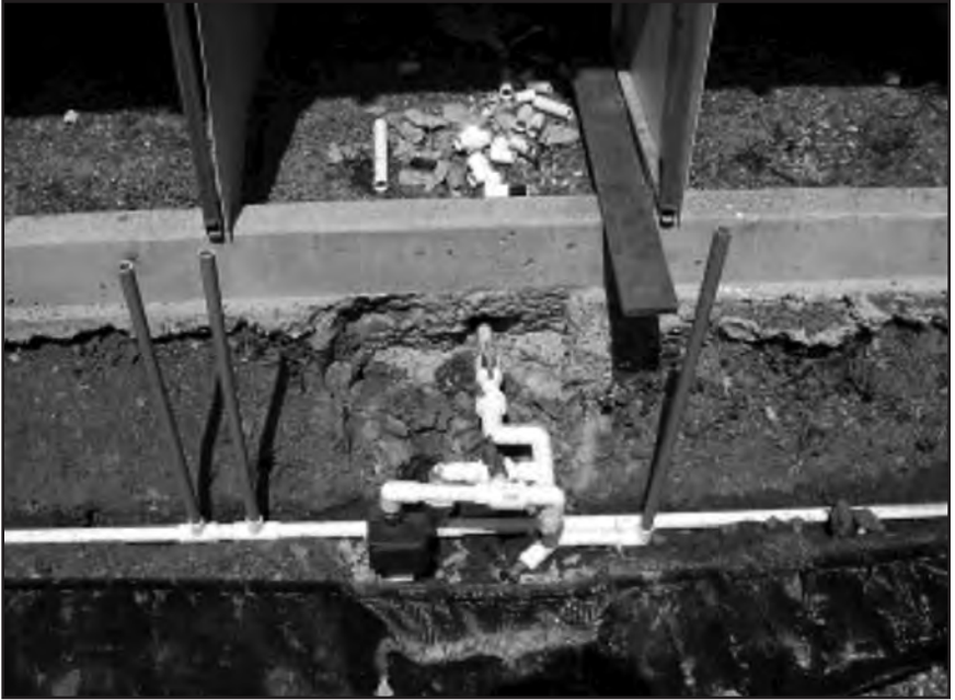
Picture showing the incoming water, a master shut off valve by the foundation and the battery operated timer for the mister system which is stubbed up on the right side of the picture.
