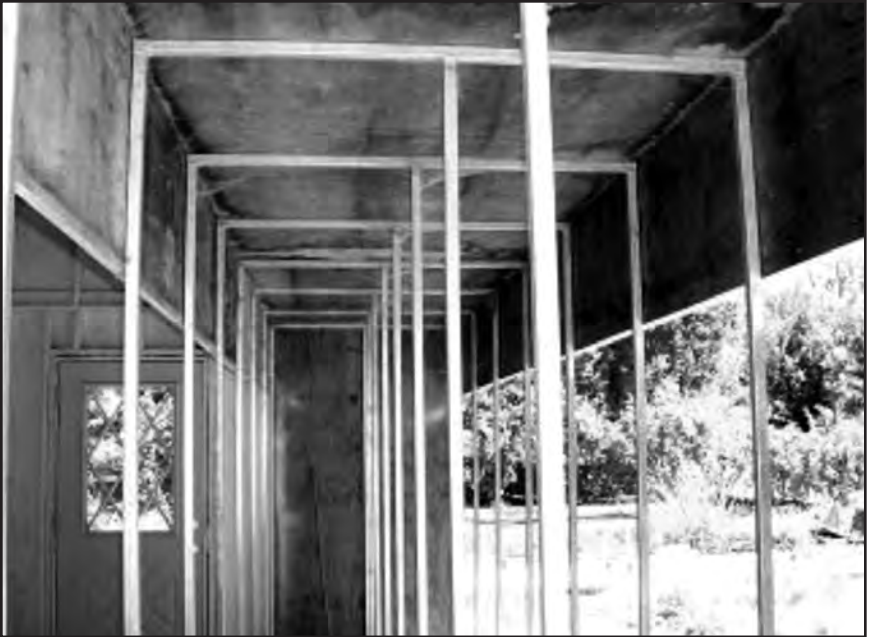
Picture showing steel frame work supporting the ceiling of the flights and above that, the roof.
