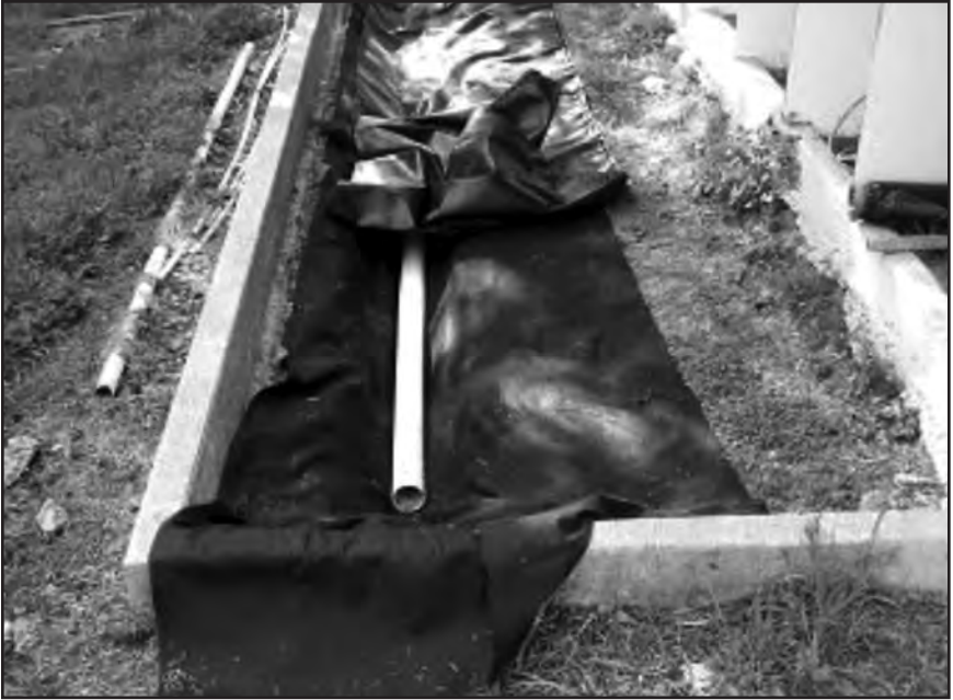
Picture showing underground drain line for outside flights. It is set in and covered with filter fabric. The fabric is used to keep the finer pieces of gravel from getting into the pipe.
