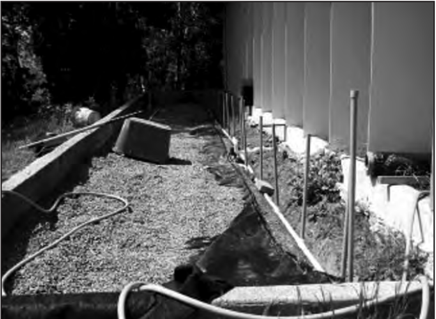
Picture showing the water main line with the services coming up at each flight. This area gets covered with gravel to within 2 of the top of the foundations.
